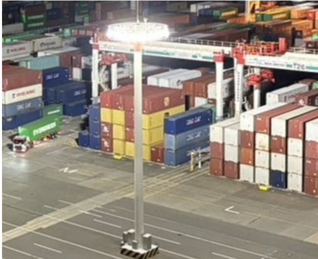
Conversion of 10 Yard Lighting Units to LED
